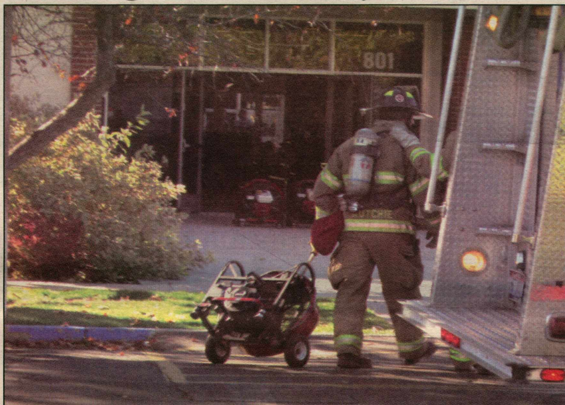
Above: Firefighters take pumps into the building to begin pumping out the standing water from the sprinklers (photo by Aimee Niles).
