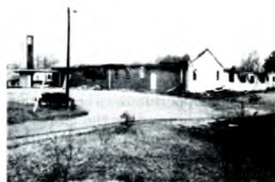
Standing walls of the Norfolk First Church were mute evidence of the total interior destruction.
