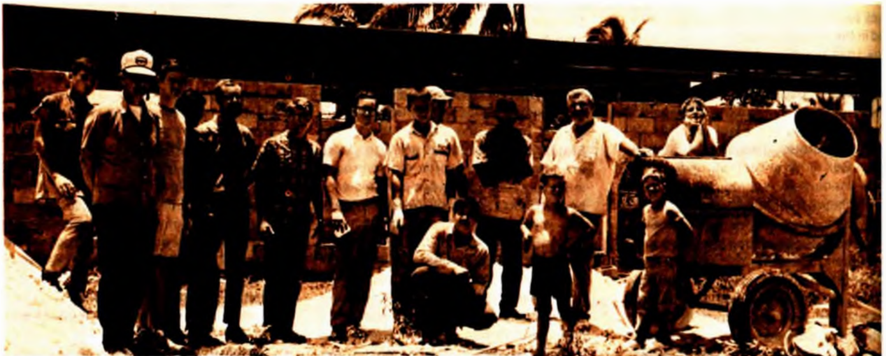
Guam Nazarene church under construction. Pastor Harold Dahlrymple stands at right with hand on the concrete mixer. Bob Wilborn contractor, is wearing a white cap. Also shown are members of the youth choir and young Guamanian Sunday school children.
